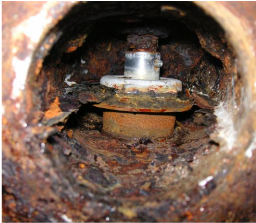
Figure 17.3.4-1: Symptom 12 - Strong corrosion in a safety valve
